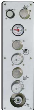
Air control panel
